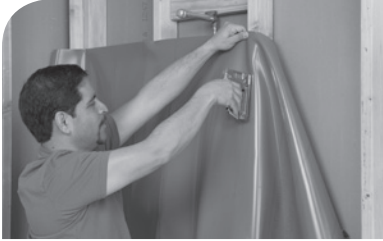
Nail or staple 16 lb roofing felt or 4 mil polyethylene sheeting to studs.
